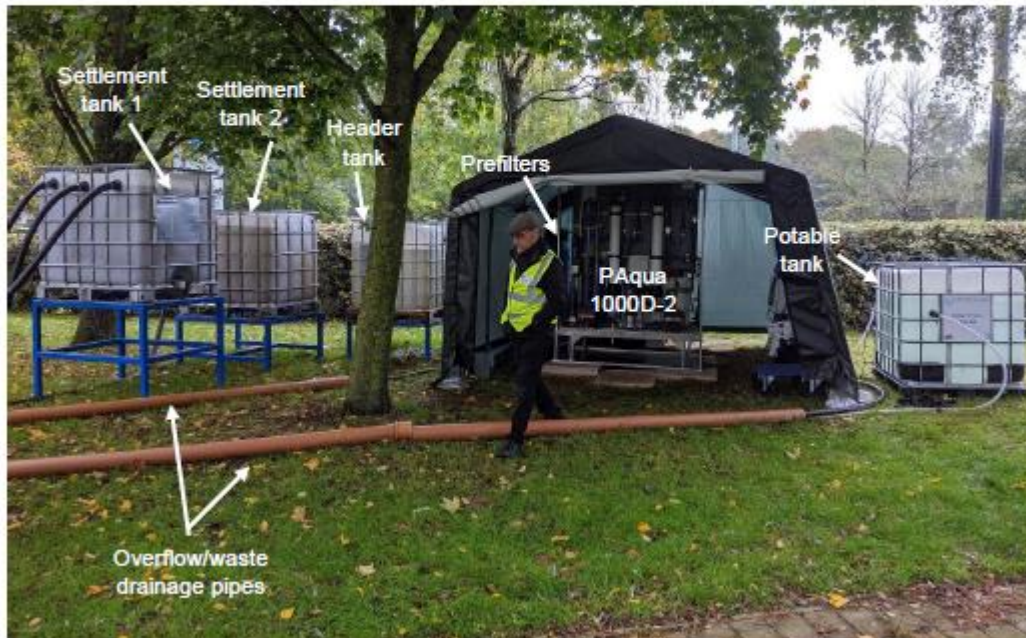
Figure 3: Picture of the NINJA drinking water treatment platform with labels to indicate the location of the PAqua 1000D-2 and the ancillary equipment. Installation on Frenchay Campus, UWE, Bristol (N51°29'56", W2°32'39").
